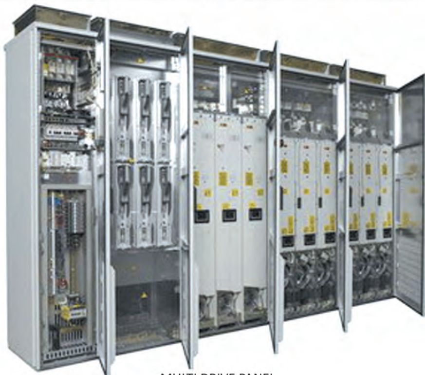
MULTI DRIVE PANEL
